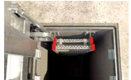
Stormwater overflow tank manholes
