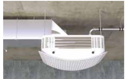
Air conditioning units
